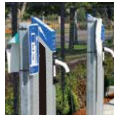
DC charging station
